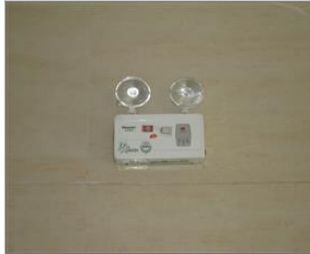
Photo of the canteen (if applicable) Emergency lighting at the canteen.JPG
