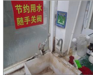
Photo of the inside of the main production hall Eye washing facility.JPG
