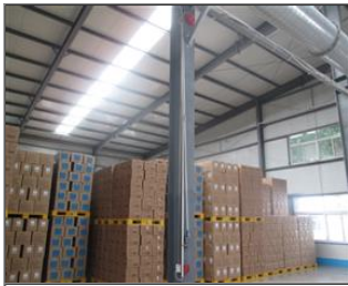
Photo of fire safety equipment Fire alarm.JPG
